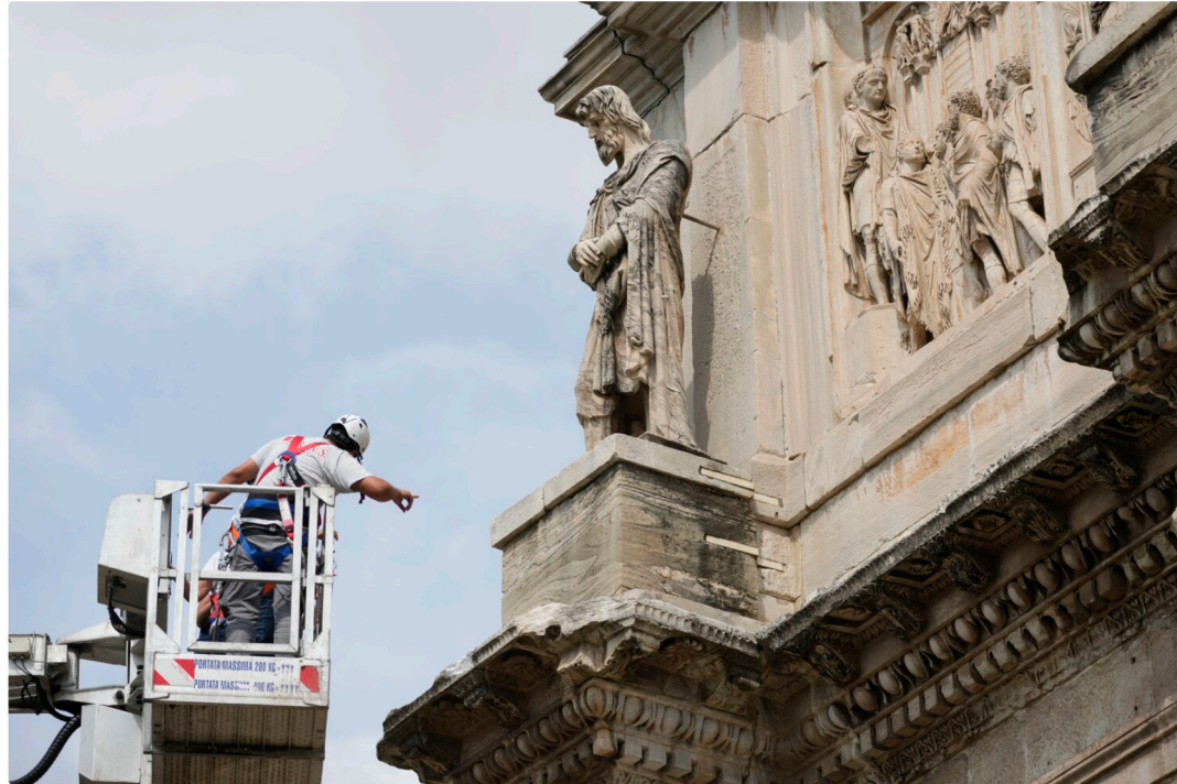
A lightning strike damages Rome's ancient Constantine Arch
